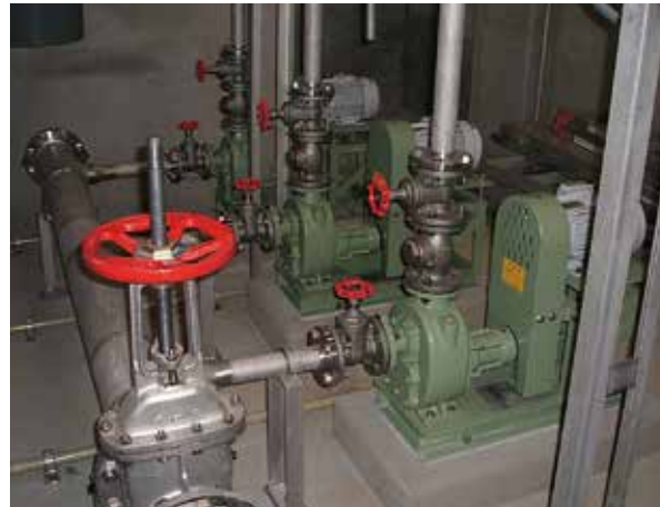
農業集落排水処理施設 汚泥引抜ポンプ Residential wastewater treatment facility Sludge withdrawal pump
